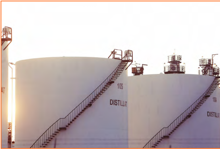
Figure 2: Typical cylindrical storage tanks.
