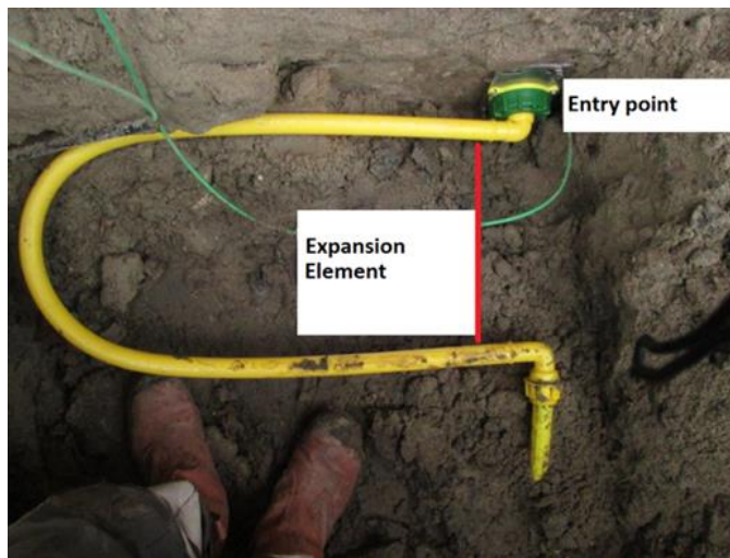
Figure 2-5: Flexible pipe connection at entry to a house (courtesy Stedin).
