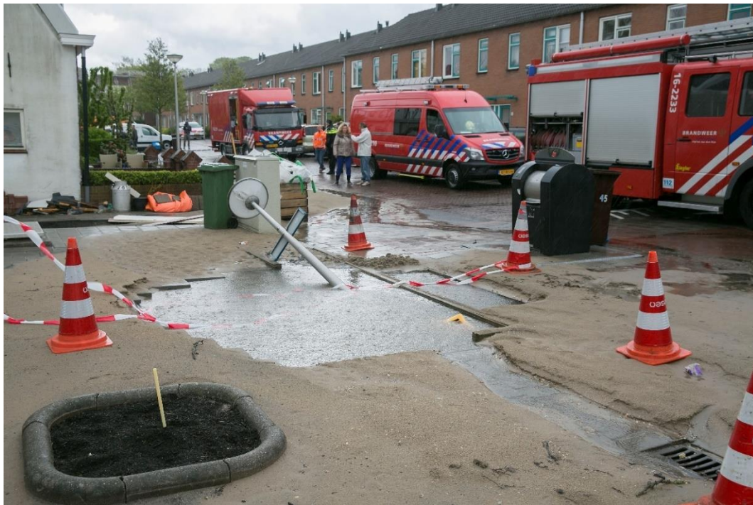
Figure 2-6: Fractured water pipe (courtesy of Oasen).
