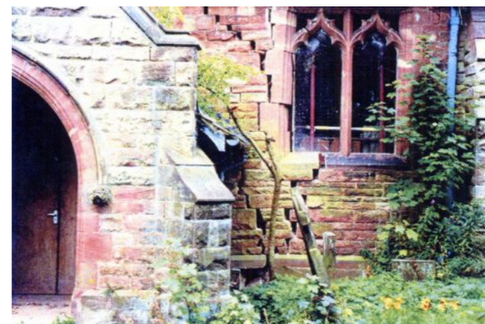
Photo A: Damage to Barlaston Church to the south of Stoke-on-Trent caused by mining induced fault reactivation. Photo courtesy of Laurance Donnelly.
